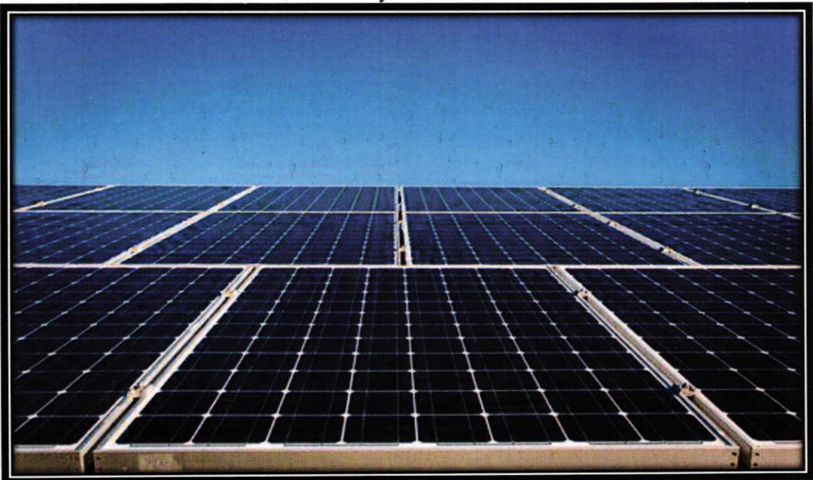
Solar PV system installed at college terrace
